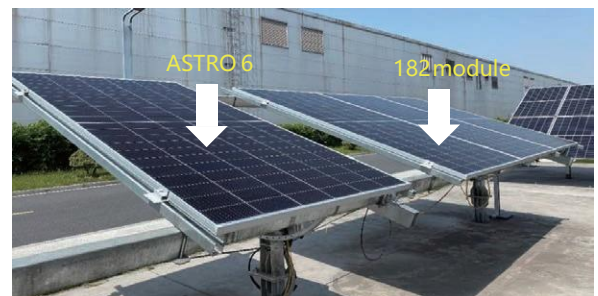
Project location: Haining, Zhejiang Province, China. Fixed tilt: 25°, ground clearance: 0.5m
